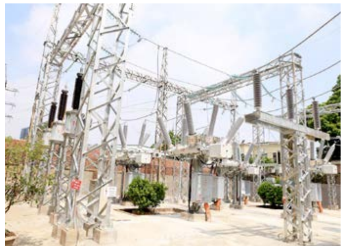
ABB PASS 145kV at Giam Substation
