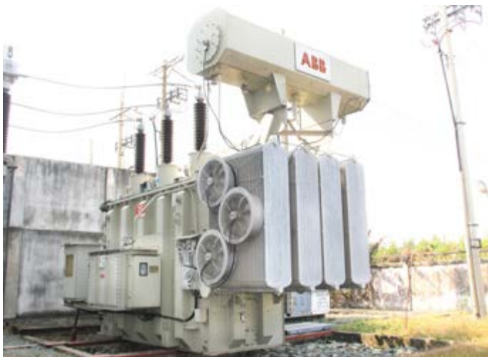
ABB Transformer at Hiep Phuoc Power Plant since 1999
