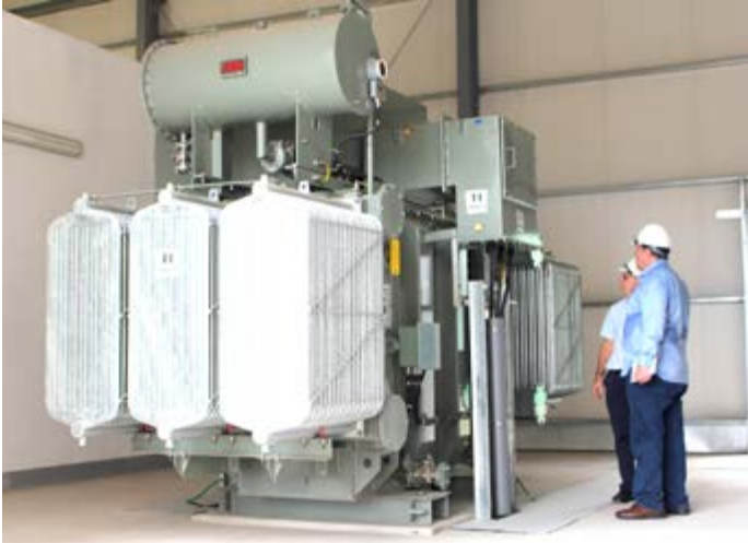
ABB Transformers at Nghe An Sugar Cogeneration Project
