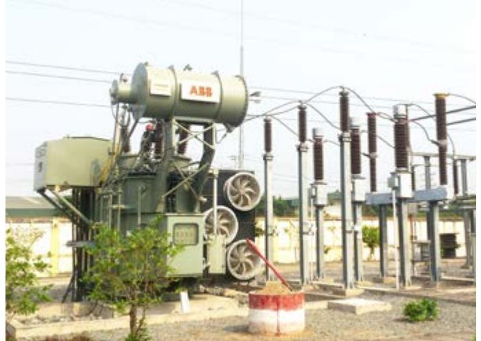
ABB at Nhon Trach 110kV substation
