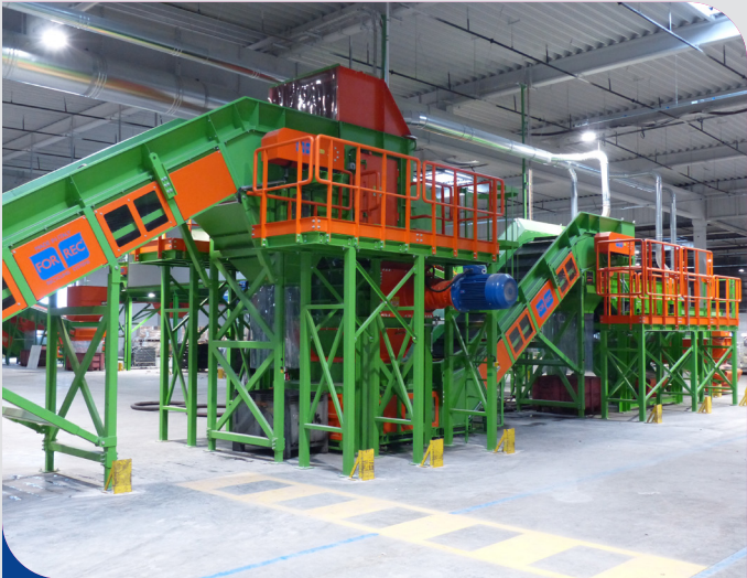
Household WEEE R4 treatment plant
