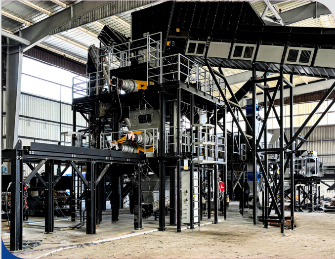
Boiler treatment plant
