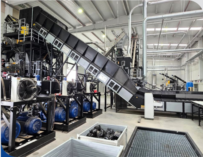
R1 treatment plant (90 units/hour)
