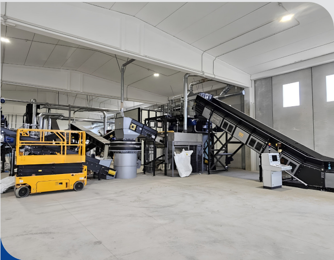
Automatic grinding and separation plant
