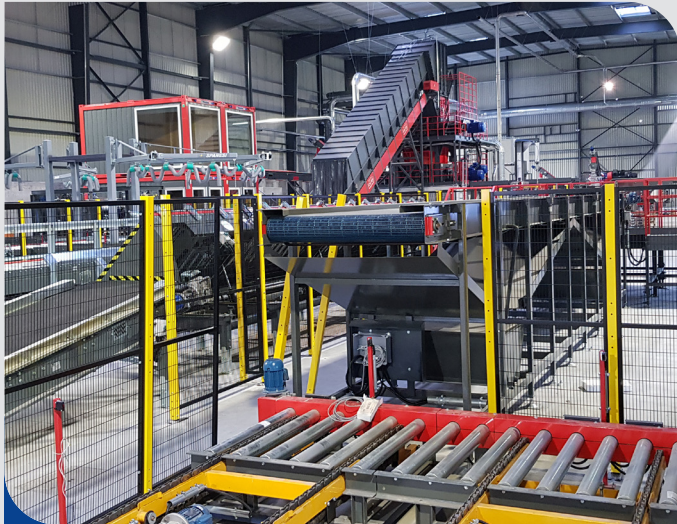
R1 treatment plant (120 units/hour)
