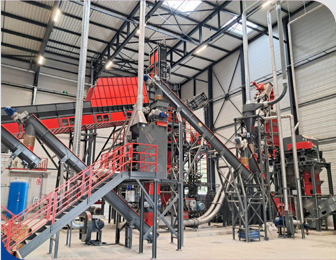
Boiler treatment plant
