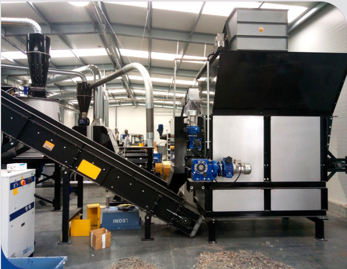
Automatic grinding and separation plant
