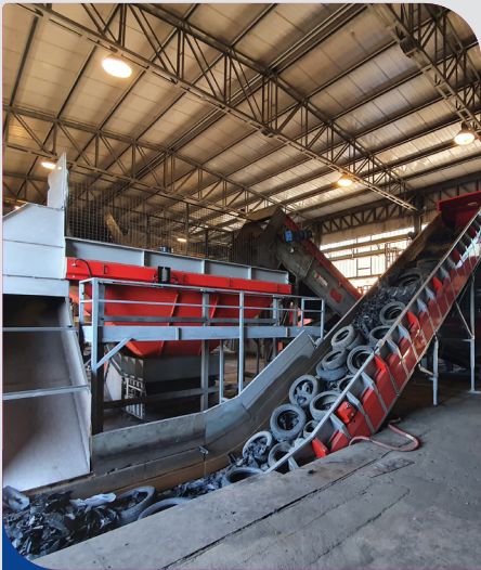
Granule production plant (< 4 mm)
