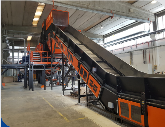
R1 treatment plant (60 units/hour)
