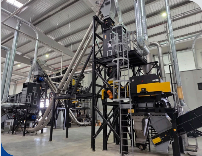
R1 treatment plant (90 units/hour)
