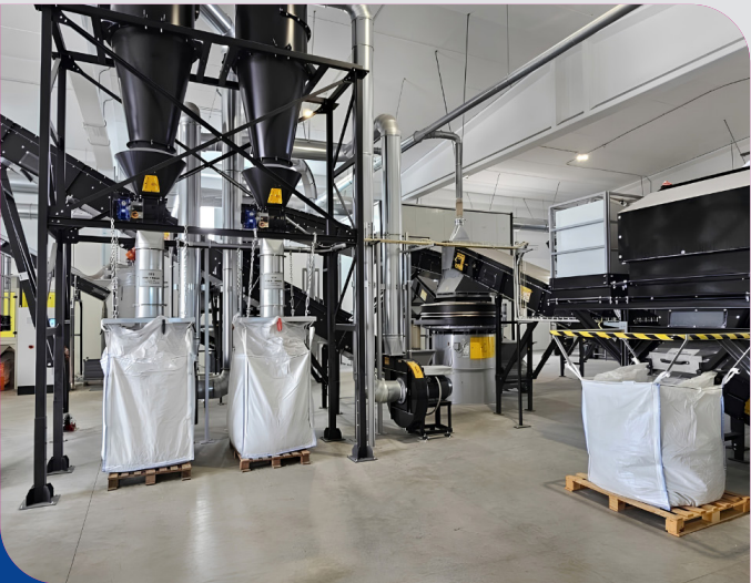
Automatic grinding and separation plant
